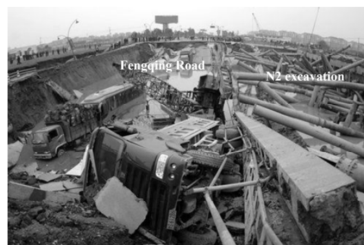
Fig. 3 View of the collapsed site for the N2 excavation
