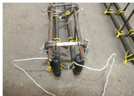
Fig. 9 Pre-wired cable of the bar
