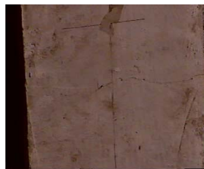
Fig.4 Crack after a stable failure
