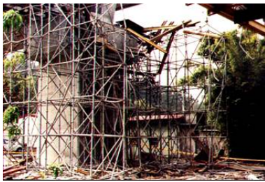
Fig.1 Collapse of system scaffolds at construction sites in Taiwan
