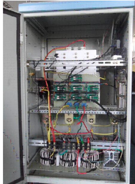
Fig. 8 Photograph of the three-level grid-connected inverter
